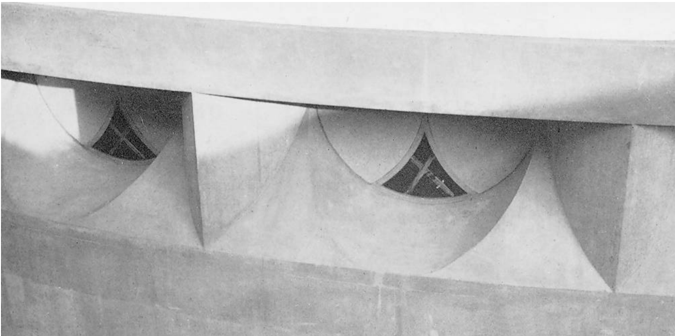
The view above shows some of the intricate precision formwork at the windows of the basement-level lecture room. Since most of the concrete in the structure is exposed, elaborate care was exercised to achieve the utmost accuracy and the finest possible surface texture.
